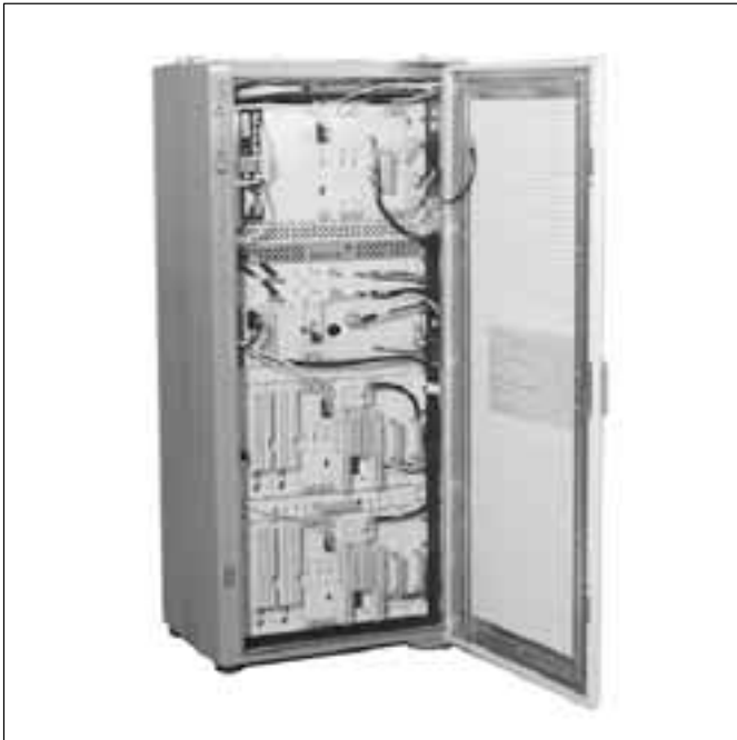
Base station of cellular network
