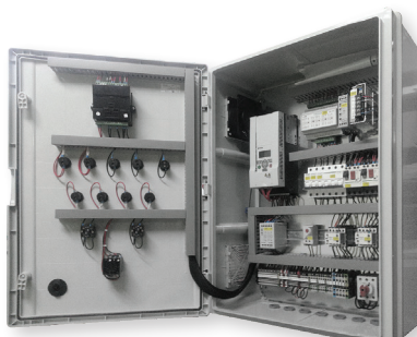
Example of control equipment and accessories installation
